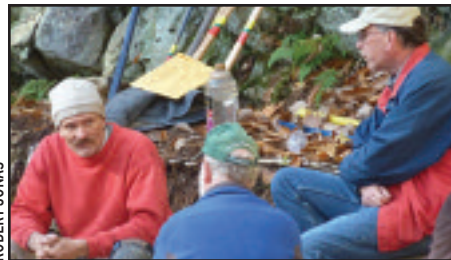
Bob Brunner, left, discusses stone work with volunteers.
