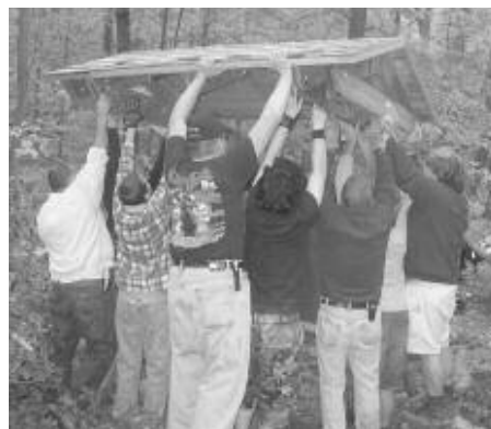
Helping hands raise the roof on an information kiosk at Norvin Green.
