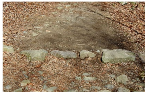
Mr. BAD BAR: The bar is running perpendicular to the trail causing water to pool behind it during wet weather.
