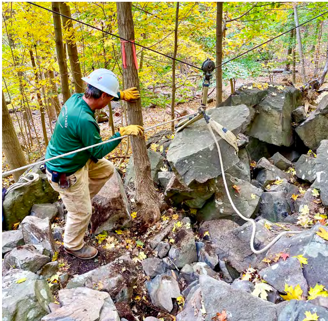
On the Upper Nyack Trail project, the Long Distance Trails Crew installed 351 stone steps, built 2,537 square feet of crib wall, and constructed 3,775 feet of sidehilled trail.
